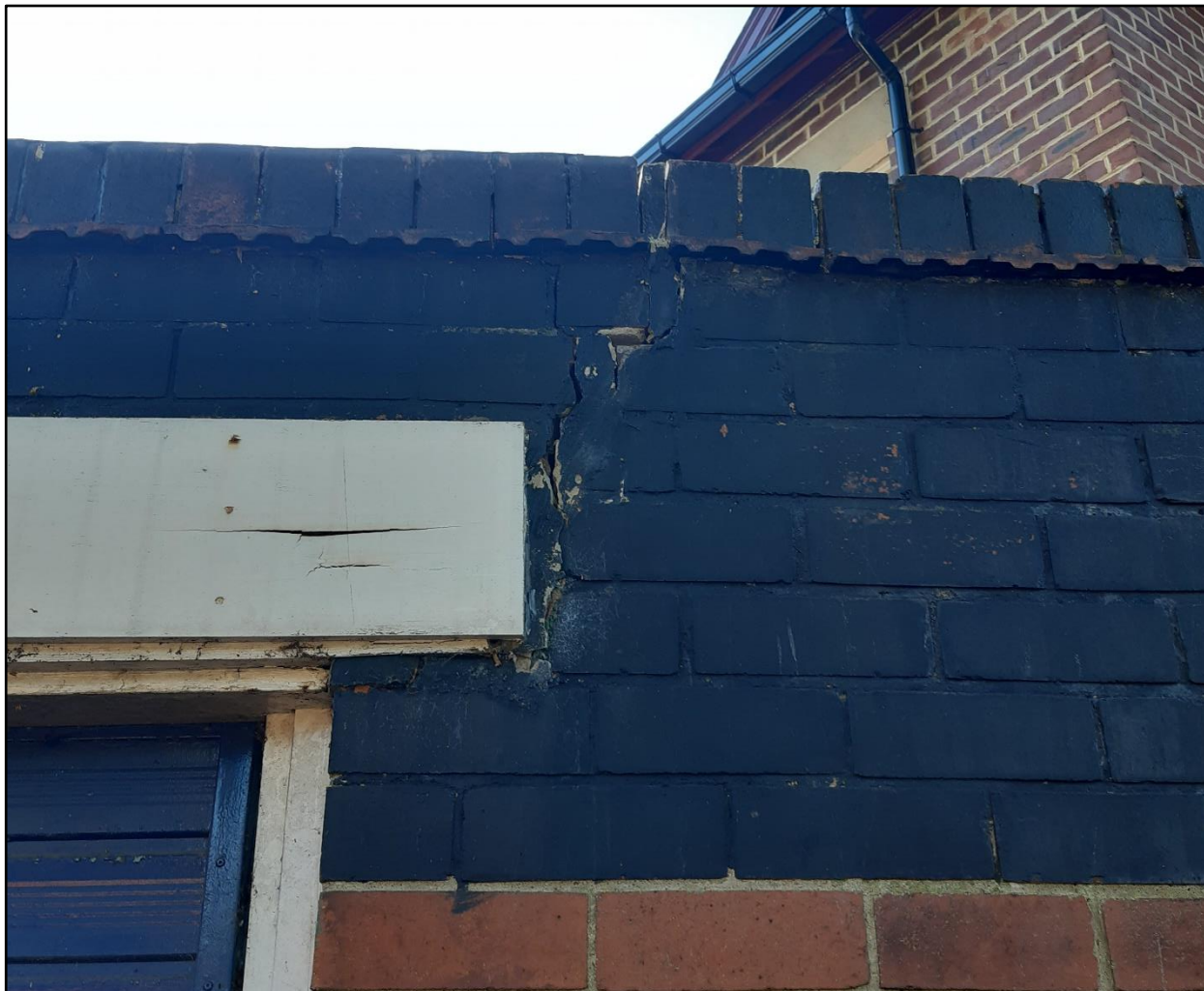
Photo 10 – Cracking adjacent to lintel on garage
